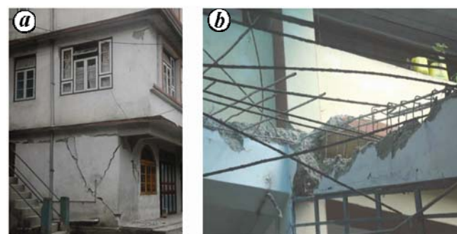
Figure 8. Damage to RC-frame buildings. a , Non-structural damage in the form of diagonal cracks in the infill walls and separation from RC frame. b , Severe structural damage to multi-storeyed, engineered school building.
