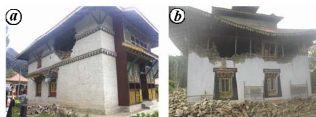
Figure 7. Extensive damage to stone masonry walls of tall heritage structures. a , Dubdi monastery, Yuksam, West Sikkim. b , Ringhim monastery, Mangan, North Sikkim.
