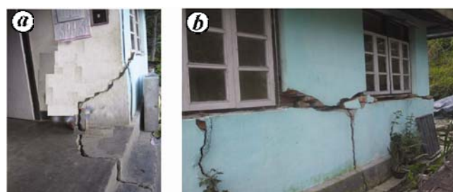
Figure 6. Damage to brick masonry houses with CGI sheet roofs. a , Subsidence due to sinking of the fill part of the foundation. b , Cracks extending up to the plinth, indicating the need for plinth beam to hold the structure together.
